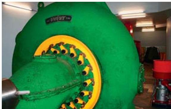
Isolation an Turbine
